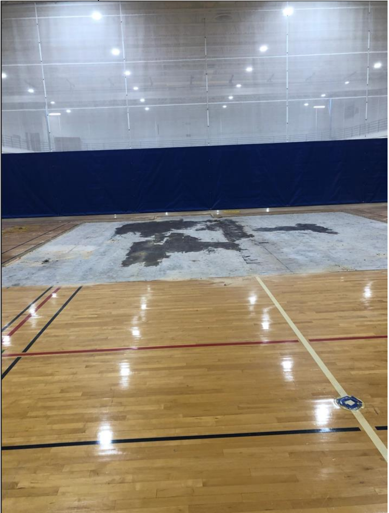
Photo of area in need of repair:
